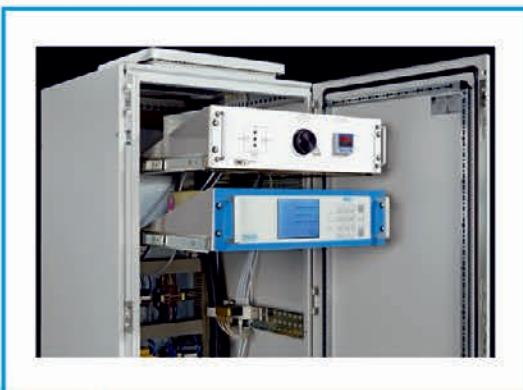
Continuous Emission Monitoring System
